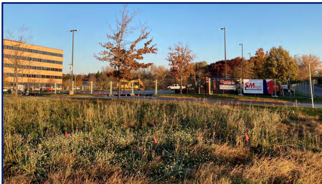
Site work for new mental health crisis center at the Dakota County Northern Service Center. Source: LOCi Consulting LLC
